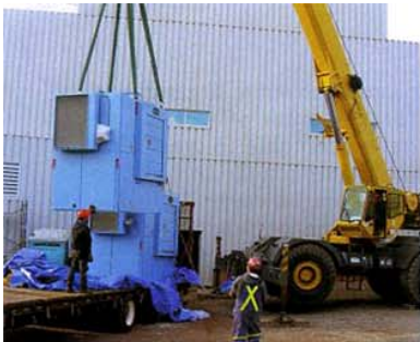
Crane lifts one of the 250-lb Braun steam dryers off the truck.
